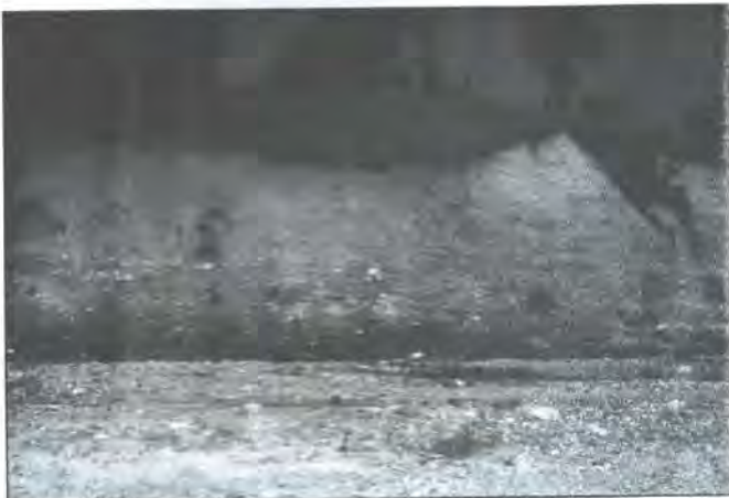
Fig. 6: A typical example of riverbank failure problems along the Kukhreni Khola near Mayurdhap
