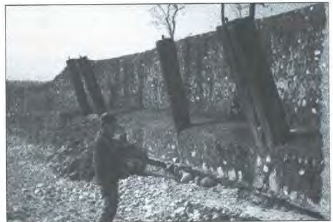
Fig. 7: Bank scouring by Kukhreni Khola, boundary wall of Hetauda Cement Factory.
