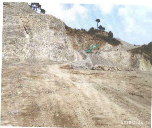
Photo 3: Vertical slopes of the Bishokarma Mines and Minerals Pvt Ltd quarry area, Dang
