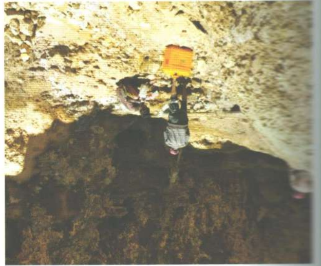
Photo 7: Salt encrustation in the conglomerate cover, the dome is within the cave-shaving fractured limestone, right side of Nursing Khola
