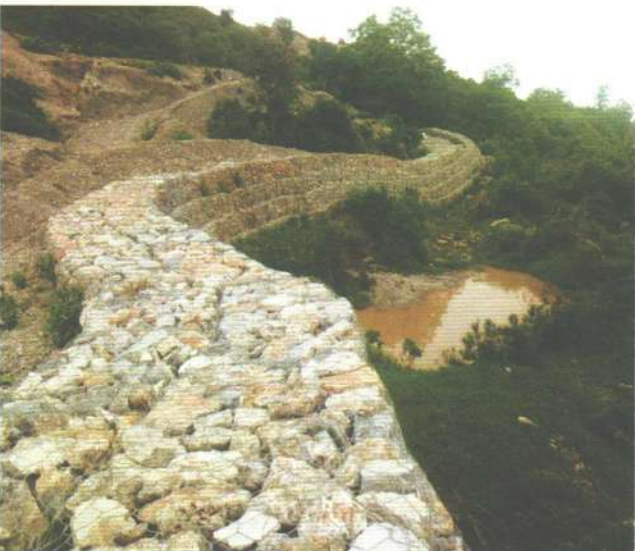
Photo 5: Check dam and siltation pond developed in basal part of the Siddhartha Minerals quarry area
