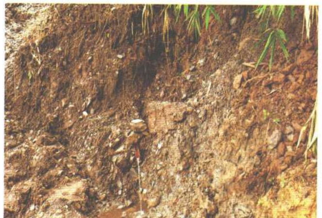
Figure 11: Water seepage at Kuraha.
