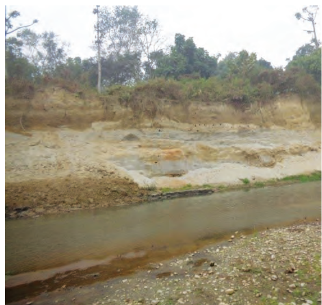
Photo 6: River bank cut prone area
